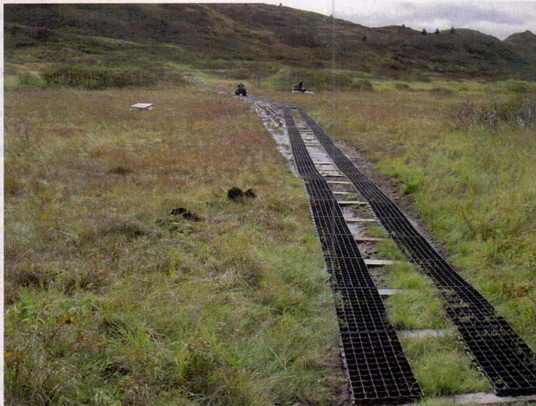
Photo 1. Typical layout of GeoBlock "Geotrack" configuration using 2 inch thick GeoBlock panels and 5 foot wide pressure treated 2X6s as cross ties. This section is installed along a new alignment of the trail. The panels are attached to the cross ties with 1 5/8" long deck screws. Utilizing this approach, only two GeoBlock panels are required for every meter of trail verses three panels for the more common full panel width configuration. This method promises to be a highly effective trail hardening method across a wide range of application sites in Alaska.
