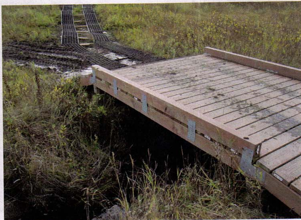
Photo 7. Typical bridge. Four 4X8s are used as underlying stringers. These are decked with pressure treated 2X6s. Additional 4X8s are used as curb rail. Short 2-3 foot ramps are also constructed out of 4X8s and 2X6 decking. The structure is supported by concrete pilings and additional 4X8 timbers.
