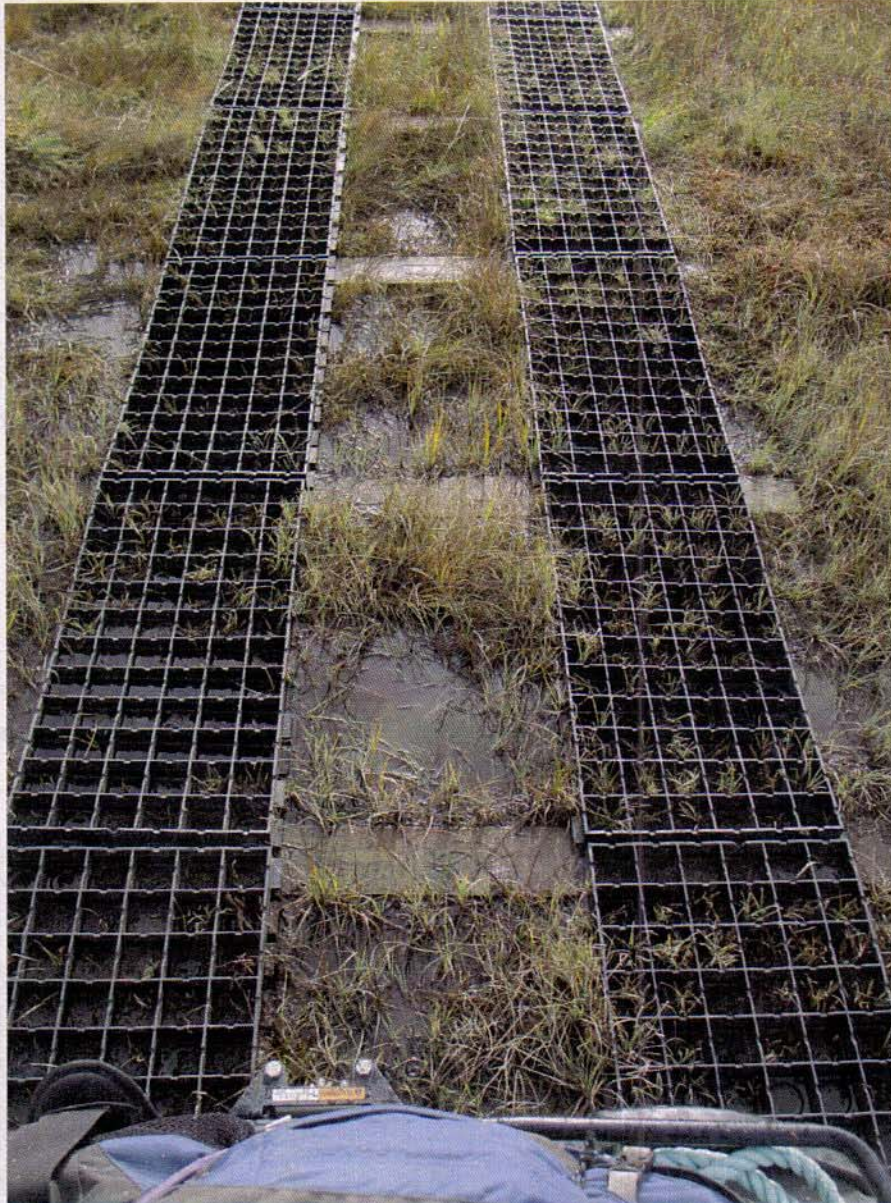
Photo 3. Closeup detail of the GeoTrack configuration. Note cross tie location at 1 meter interval to match length of GeoBlock panels. Note also, the 6 inch inset of the panels on the 6 foot long cross ties resulting in a 5 foot wide tread. At this site little grubbing was required to embed the cross ties. That may not be the case at other locations so labor costs could increase.
